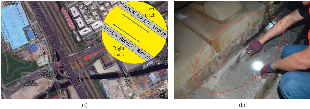
FIGURE 8: Monitoring site: (a) Site location; (b) Repair work of the L00526 track plate.
